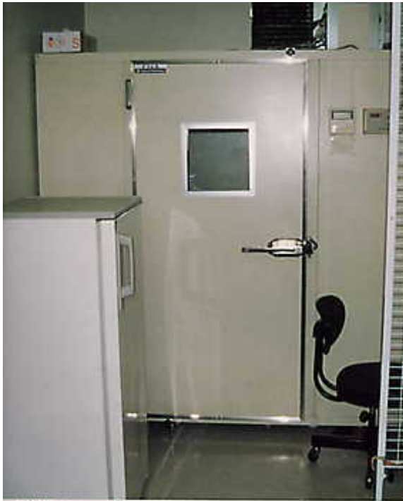
▲冷蔵室 / Refrigeration room
